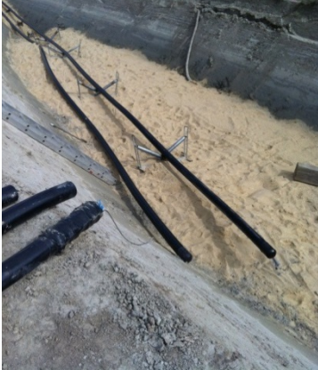
Figure 20 Cable ends in jointing pit
