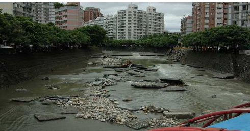
Dike failure in 2008 TP Kalmaegi
