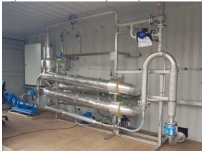
Figure 4-5 Torwash system (Source: TNO)
