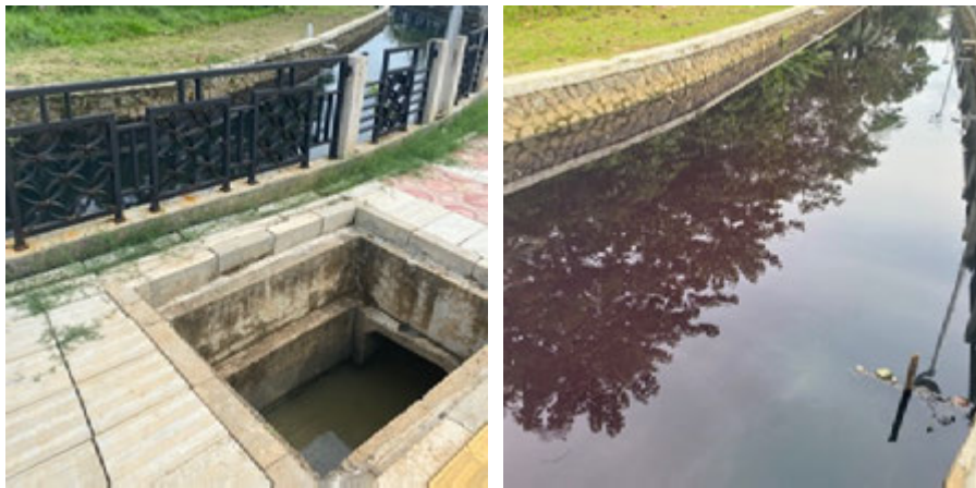
Figure 23 Unused Simbang Kulon WWTP makes river contaminated by wastewater
