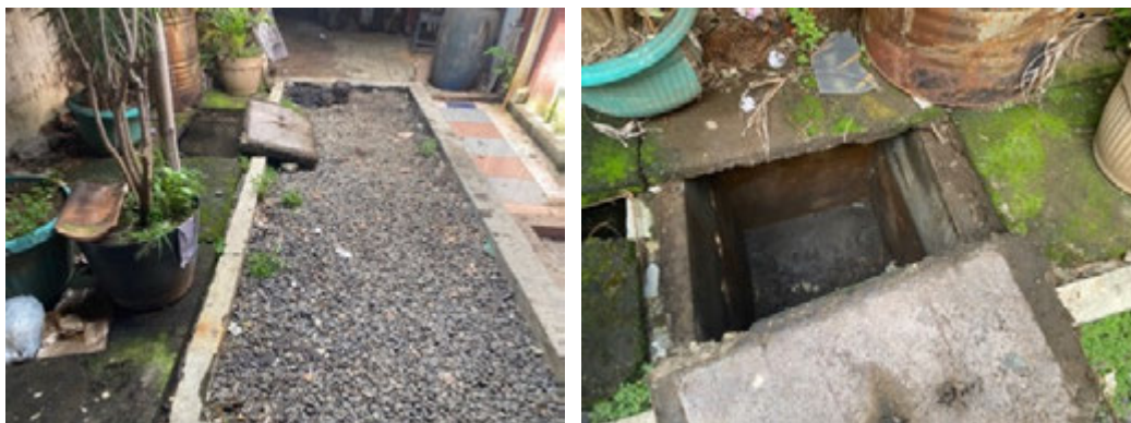
Figure 18 Individual WWTP in Batik Larissa
