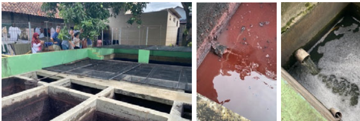
Figure 19 Kauman Communal WWTP (left), the batik wastewater (middle), the discharge water from the WWTP (left)
