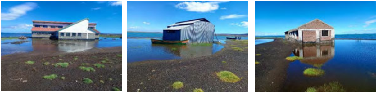
FIGURE 15 STRUCTURES RELATED TO THE FISHING INDUSTRY IN LOIYANGALANI (MARSABIT COUNTY) FLOODED DURING THE RECENT HIGH WATER LEVELS IN LAKE TURKANA. THE PROCESSING FACTORY TO THE LEFT IS 3 YEARS OLD BUT HAS NEVER BEEN PUT INTO OPERATION DUE TO LACK OF FRESH WATER. PHOTOS TAKEN IN NOVEMBER 2023 BY ABDULKAREEM ABDI.
