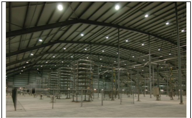
Afb. 2.29: Condensatoren in de Filterhal
