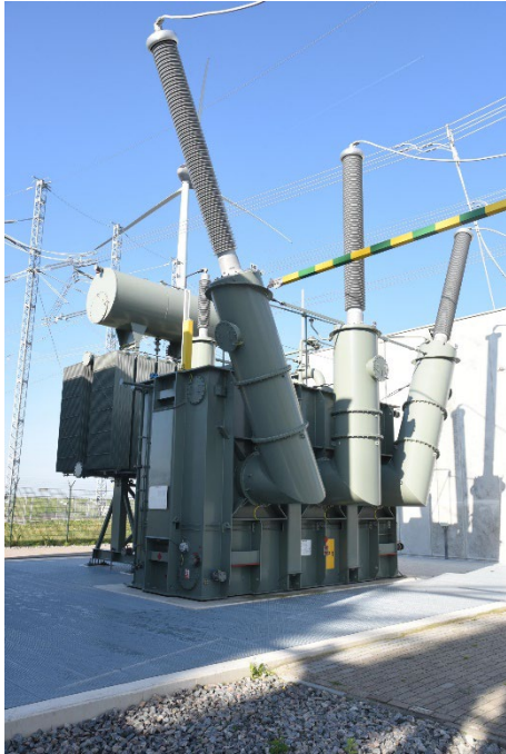
Figure 14: Example of a 380 kV reactor with a rating of 150 Mvar
