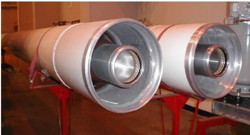
Figure 17: Inside view of a GIL (GE)
