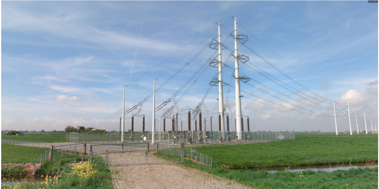
Figure 15: Overhead line - cable transition point, double circuit (connection Bleiswijk - Vijfhuizen 380 kV, Wintrack towers)
