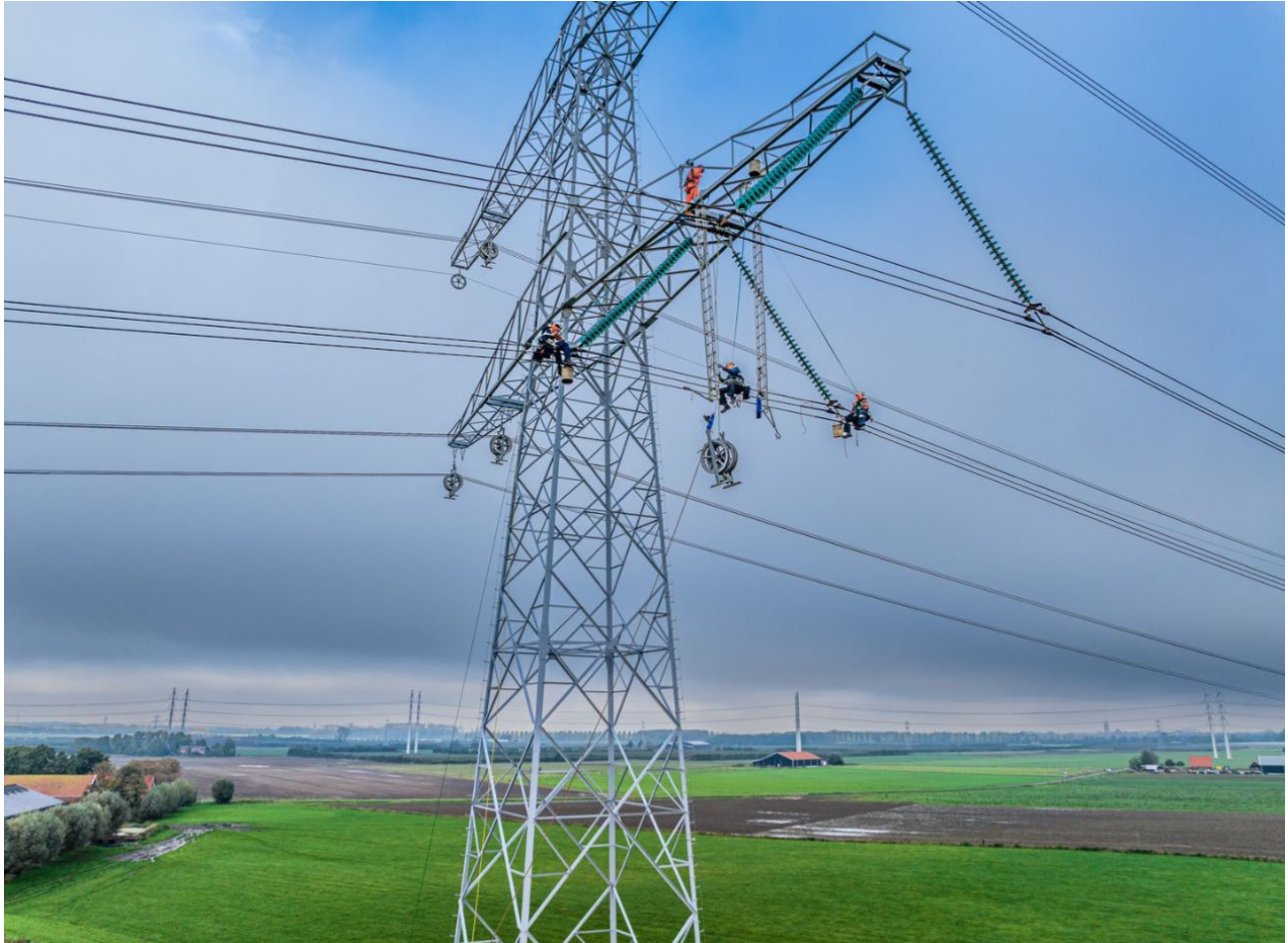
Figuur 5.4: Ophangen isolatoren of isolatorkettingen
