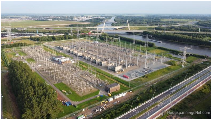
Figure 8-2 Example of a 380/150 kV substation (Diemen)
