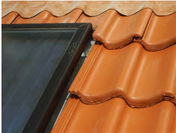
Figure 106: Top of the installed PVT panel
