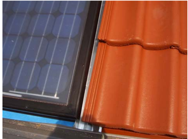
Figure 107: Bottom of the installed PVT panel
